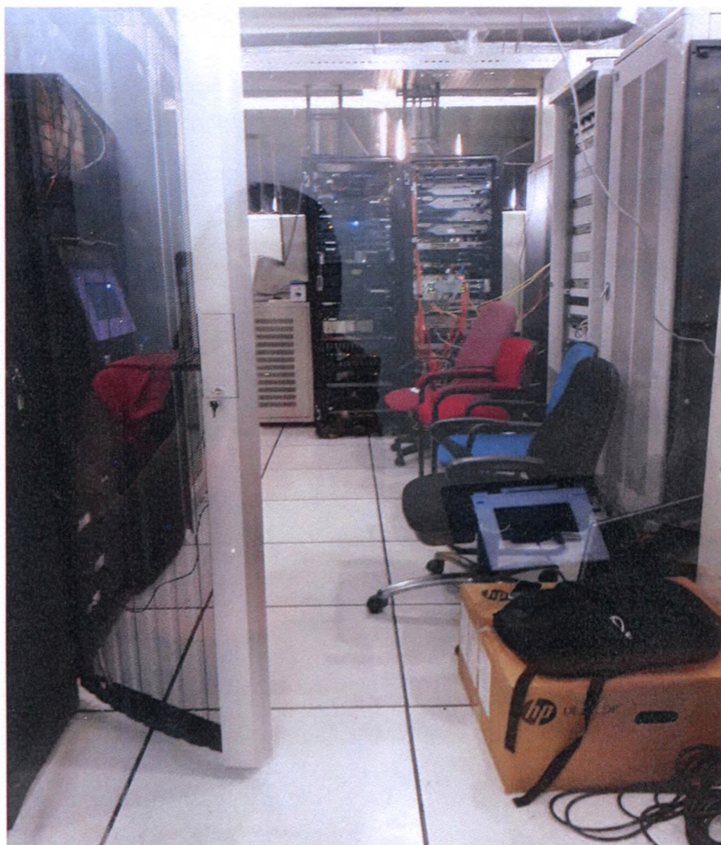
Server room in DMC
